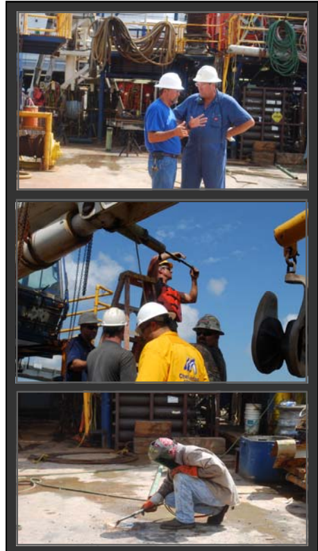
Crews ready the DSV Joanne Morrison for mobe out to perform work on two subsea wells.
